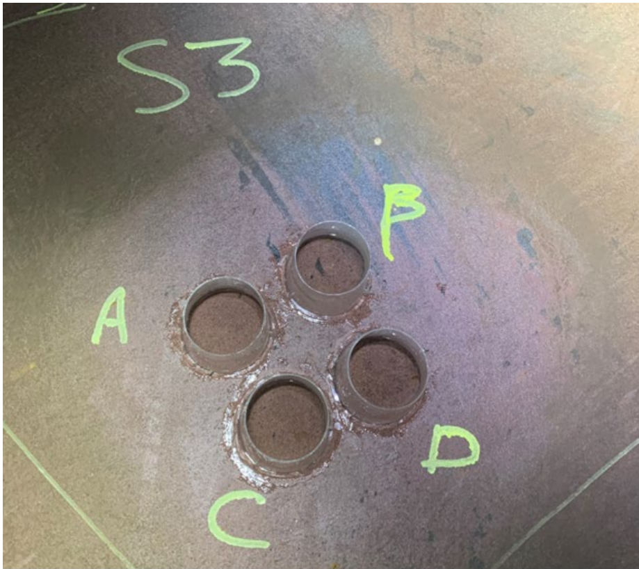
Figure 4. Visual assessment of VR3 (System 5) and EIS test setup. Notice no corrosion or blisters after 70 years of service in 18-20 ft/s flowing water conditions.
