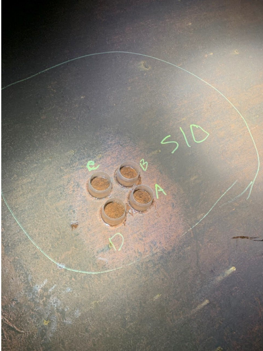
Figure 14. EIS Location 10 red lead with oil-based primer, West side of pipe. It was too difficult from photos to determine if the topcoat was System 8 or 8A.
