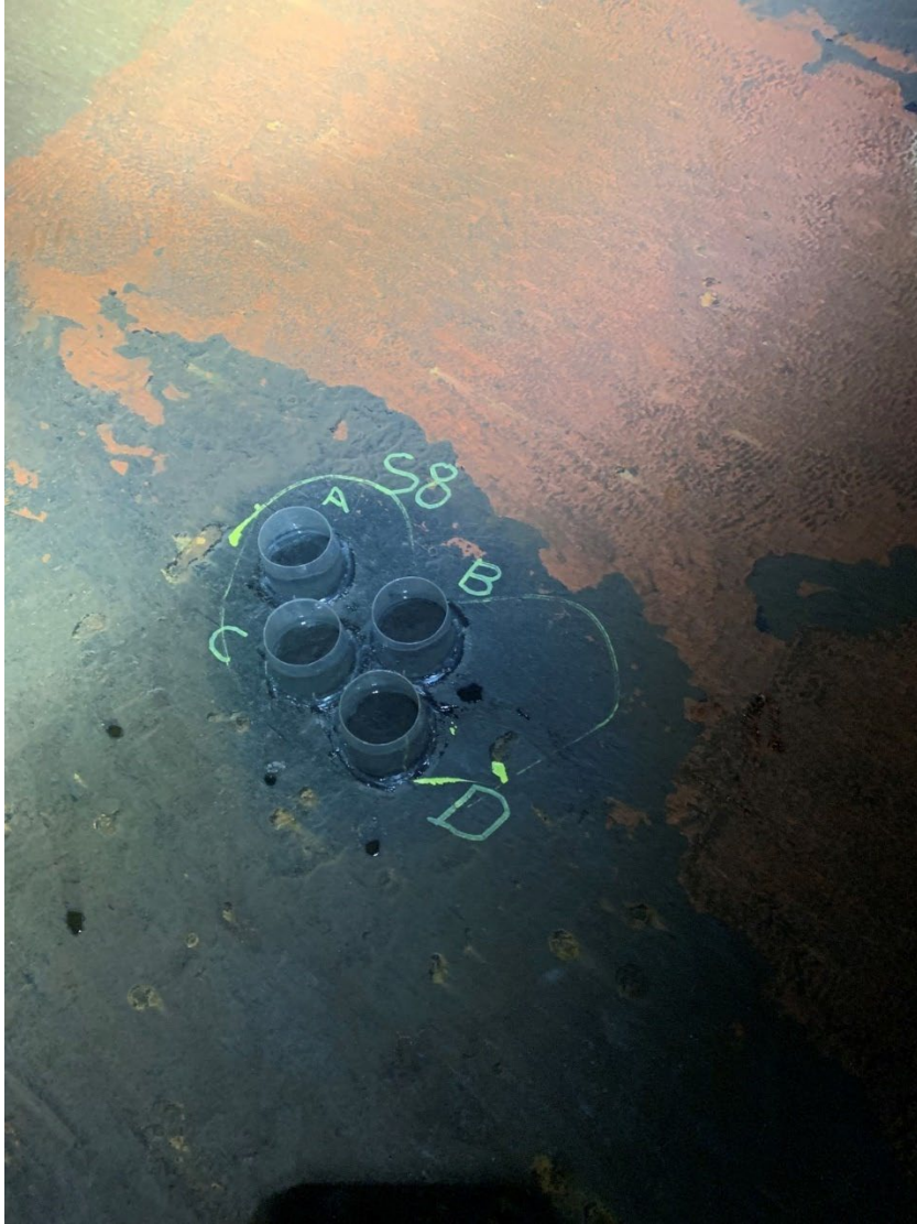
Figure 10. EIS location S8, Coal tar CA-50 (System 7) with adjacent exposed primer.
