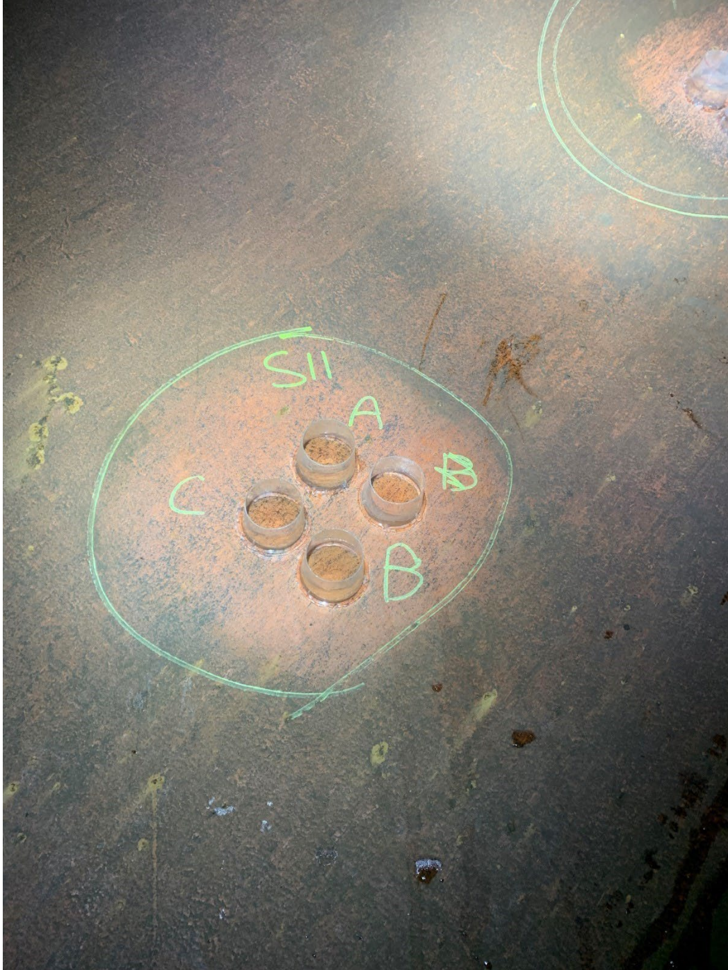
Figure 16. EIS Location 11, System 8A-1 Direct to metal
