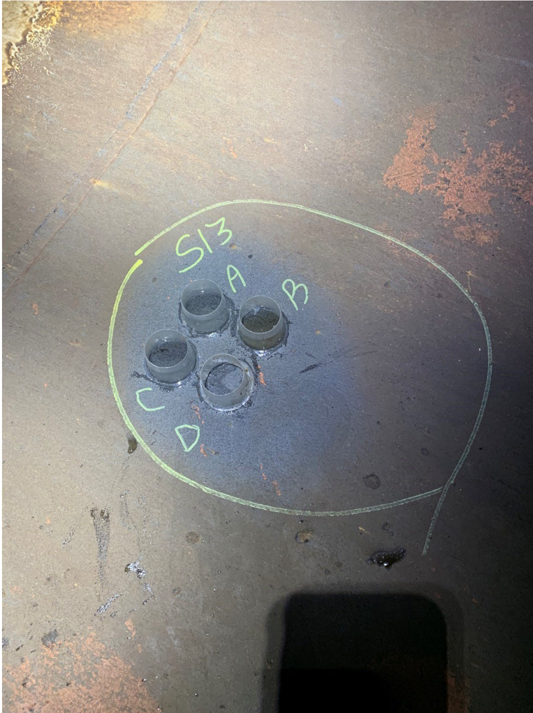
Figure 20. EIS location S13, coal tar enamel with lead-based primer
