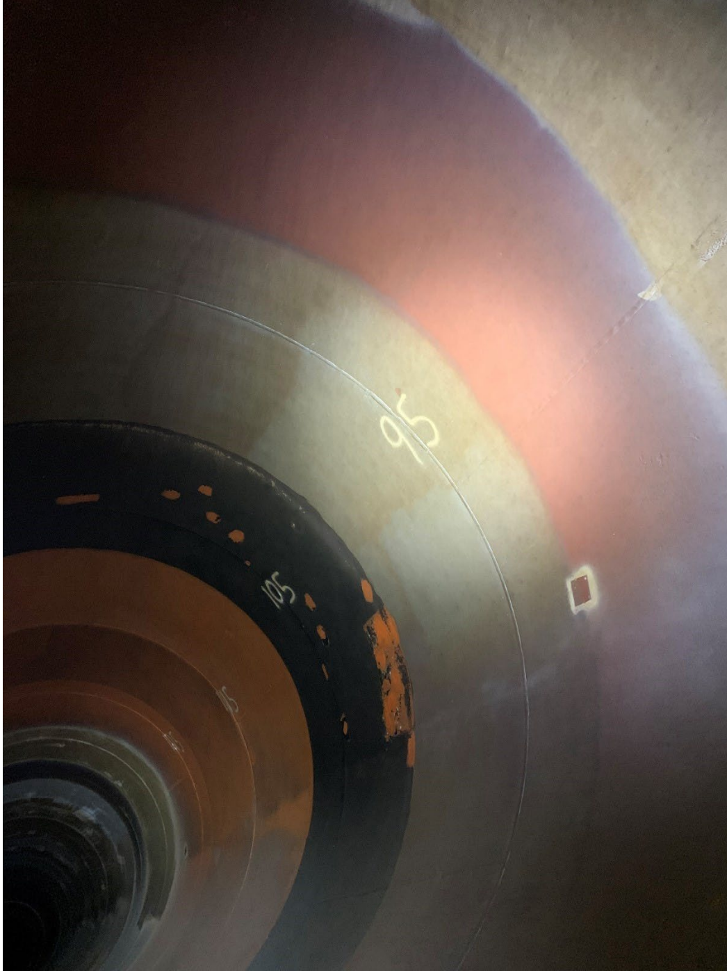
Figure 3. Visual condition of all test systems 5-8. Red lining system 5 VR3, (section 95 in photo) gray lining system 6 VR 6, (section 105 in photo) black lining system 7 CA-50 or CTE with red lead primer, (between sections 115 and 125) red lead systems 8 and 8A looking down the pipe ((8-1) direct to metal, (8-2) right side (West side) oil based primer), and (8-3) left side (East side) vinyl wash primer, and moving down the pipe red lead system 8A (additionally contains chromate inhibitor pigments) (8A-3) left side (East side) vinyl wash primer, (8A-2) right side (West side) oil based primer, and, (8A-1) direct to metal)
