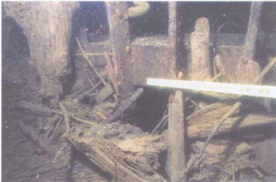
Figure 8. Photograph from Reclamation's Columbia-Pacific Northwest Underwater Inspection Team of Keechelus Dam, Yakima Project, Washington on October 27, 2005 showing woody debris and sediment build up at the base of a trashrack.
