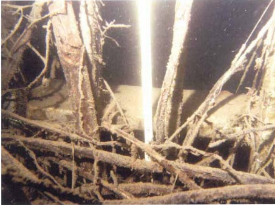
Figure 9. Photograph from Reclamation's Columbia-Pacific Northwest Underwater Inspection Team of Twin Lakes Dam, Fryingpan-Arkansas Project, Colorado on October 12, 2010 showing a two-foot high mat of twigs, sticks, and branches on the vertical trashracks of the outlet works intake structure.
