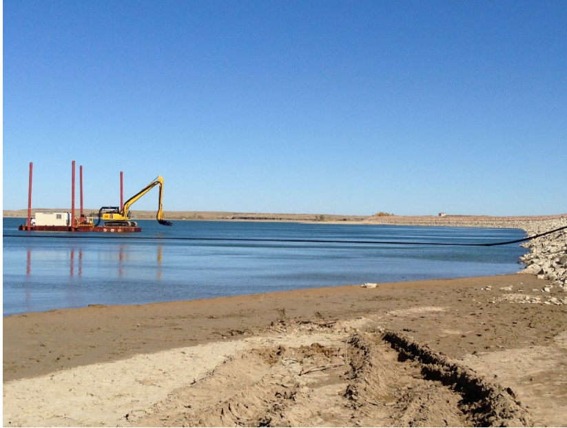
Figure 11. Sediment dredging has occurred twice in the reservoir at Belle Fourche Dam around the South Canal intake. Woody debris collected along the dam embankment rip rap is saw cut and hand removed.
