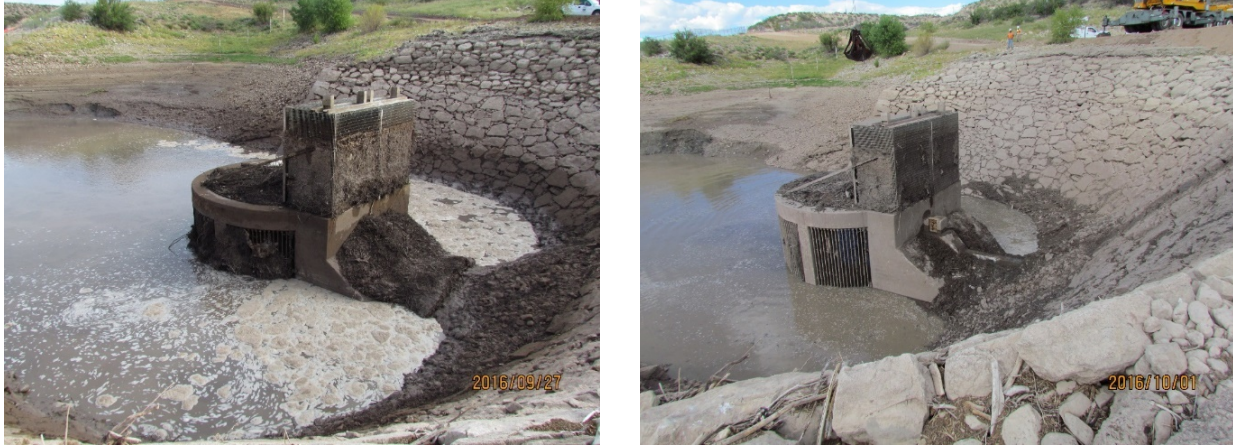
Figure 16. Caballo Dam, New Mexico before (left) and after (right) debris removal with crane and clamshell bucket. Although annual O&M costs related to debris removal are typically low, a debris clogging incident at the intake created a unique maintenance cost for contracted dredging services.
