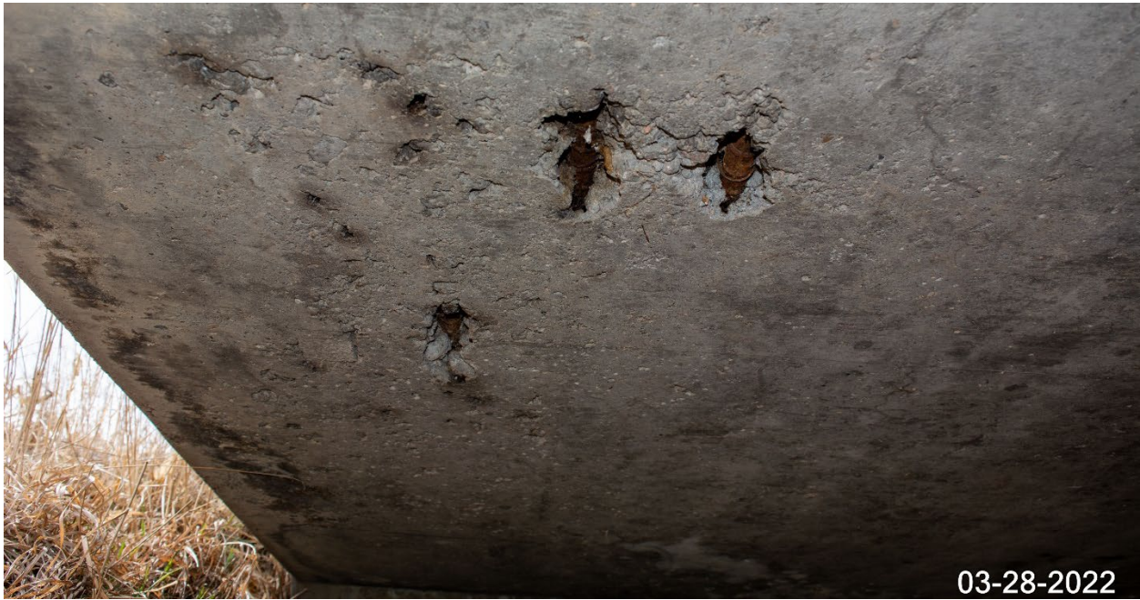
Figure B-4.—Type 1 bridge. Location noted as having exposed rebar. Corrosion is not explicitly mentioned in the inspection reports, but the rebar corrosion and concrete damage may be due to inadequate cover.
