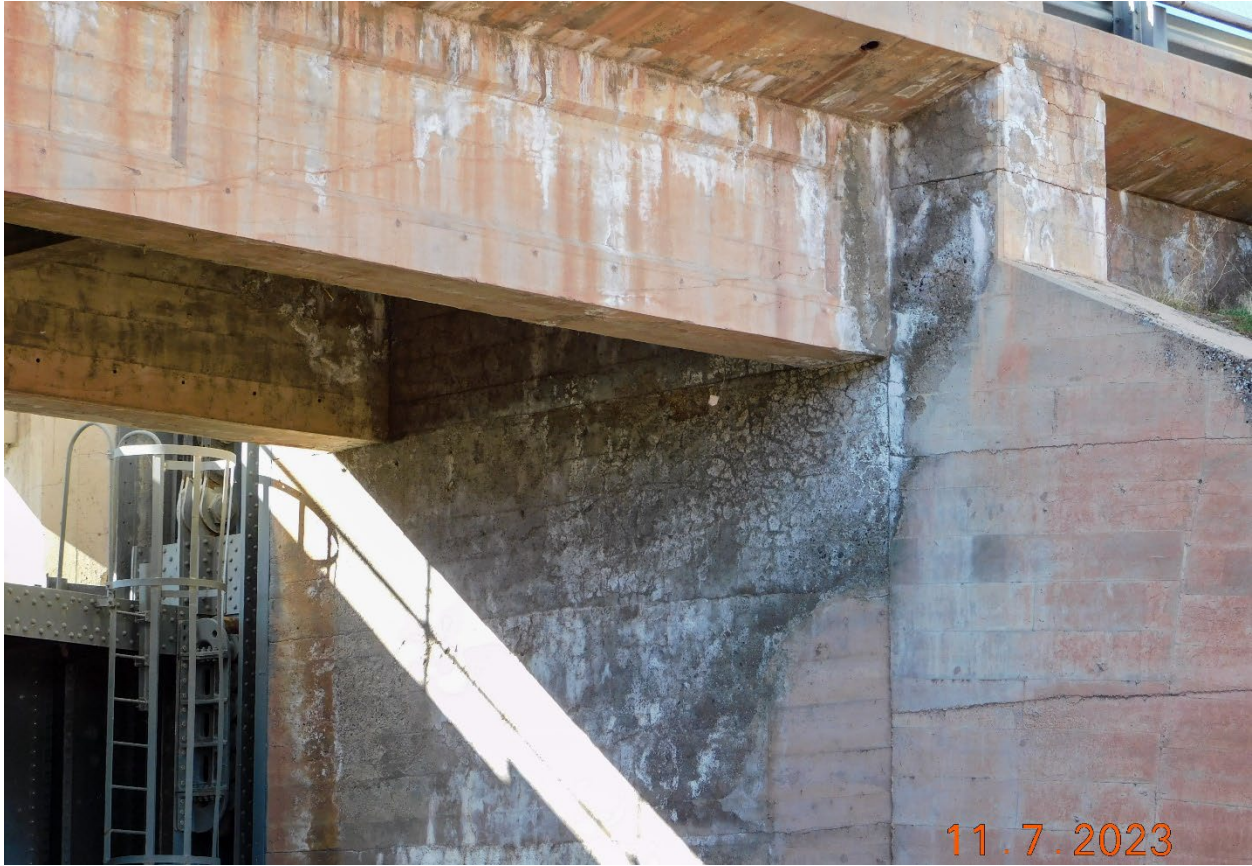
Figure B-2.—Type 1 bridge. Location noted as having deterioration, cracking, efflorescence, spall, and water staining. Corrosion was not noted as an issue.
