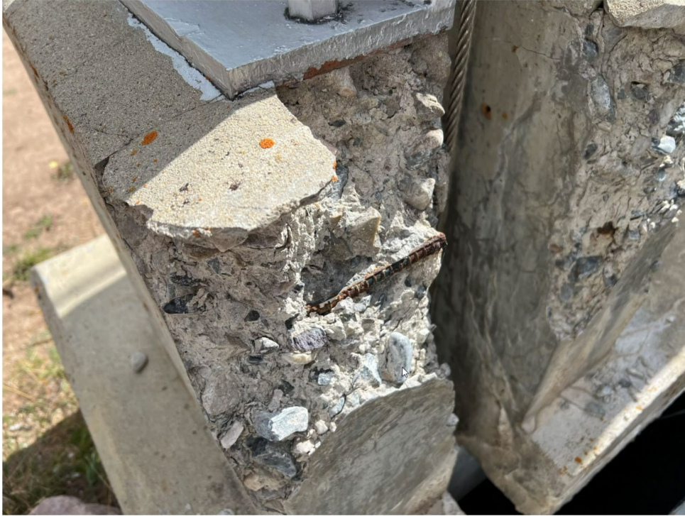
Figure A-3.—Spalling pedestal with exposed reinforcing steel. The initial cause of the concrete deterioration is unknown.
