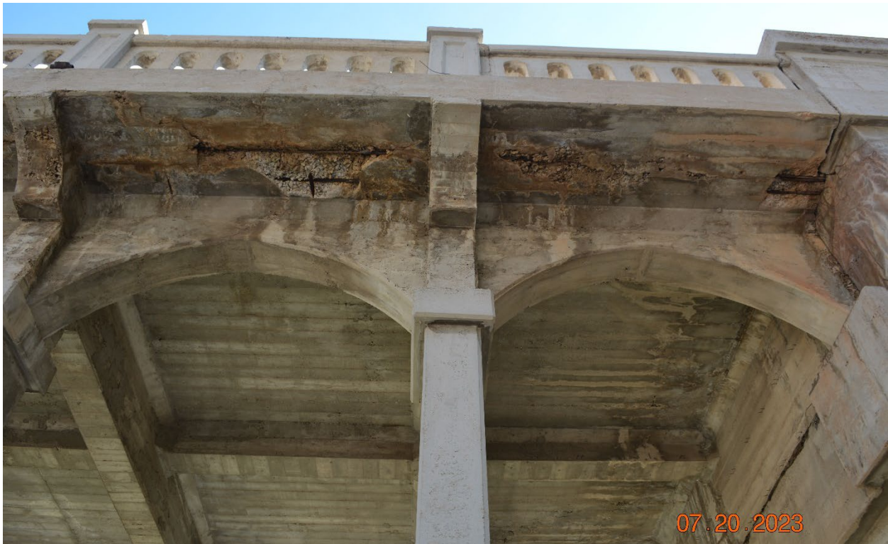
Figure B-1.—Type 1 bridge. Location noted as having deterioration, cracking, efflorescence, rust staining, spall, and exposed rebar with corrosion.
