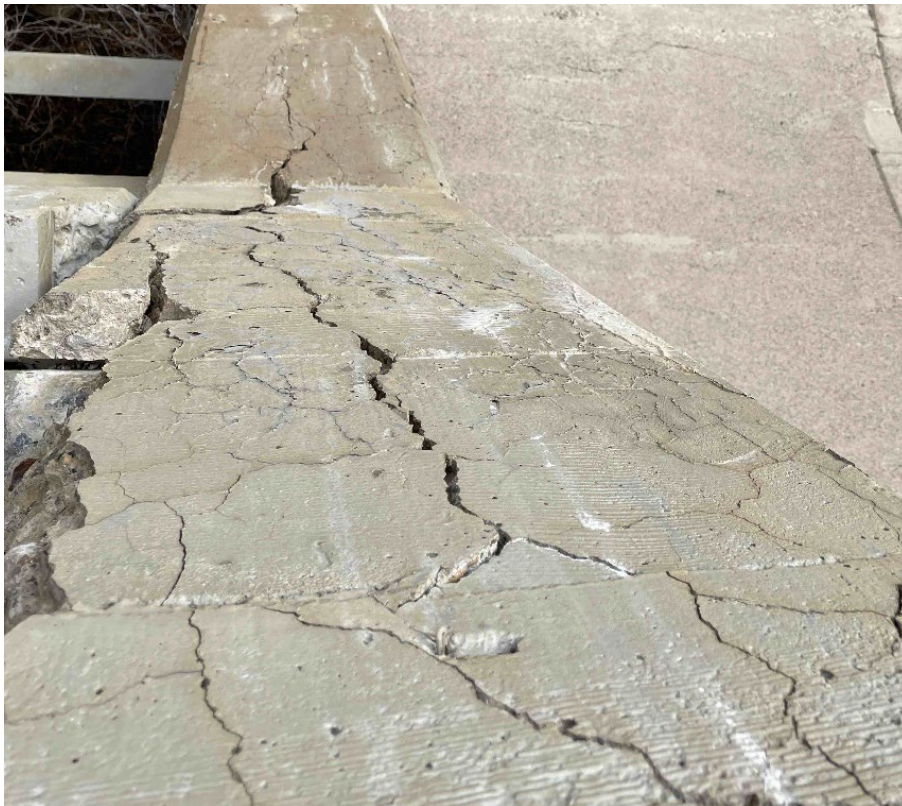
Figure A-8.—Cracking along a parapet wall due to freezing and thawing.
