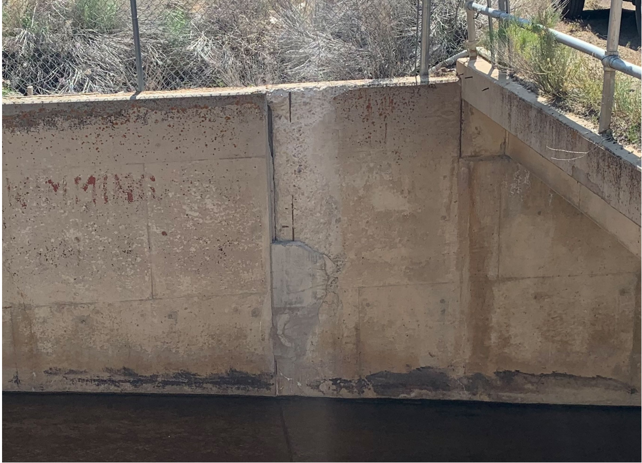
Figure A-2.—Deteriorated concrete with exposed reinforcing steel that has required multiple repairs at the same location. The suspected cause is ASR and subsequent freeze-thaw. Notes on other structures from the same region: roadways that are treated with deicing salts in the winter have not experienced major spalling or delamination, just minor cracking and a few popouts.
