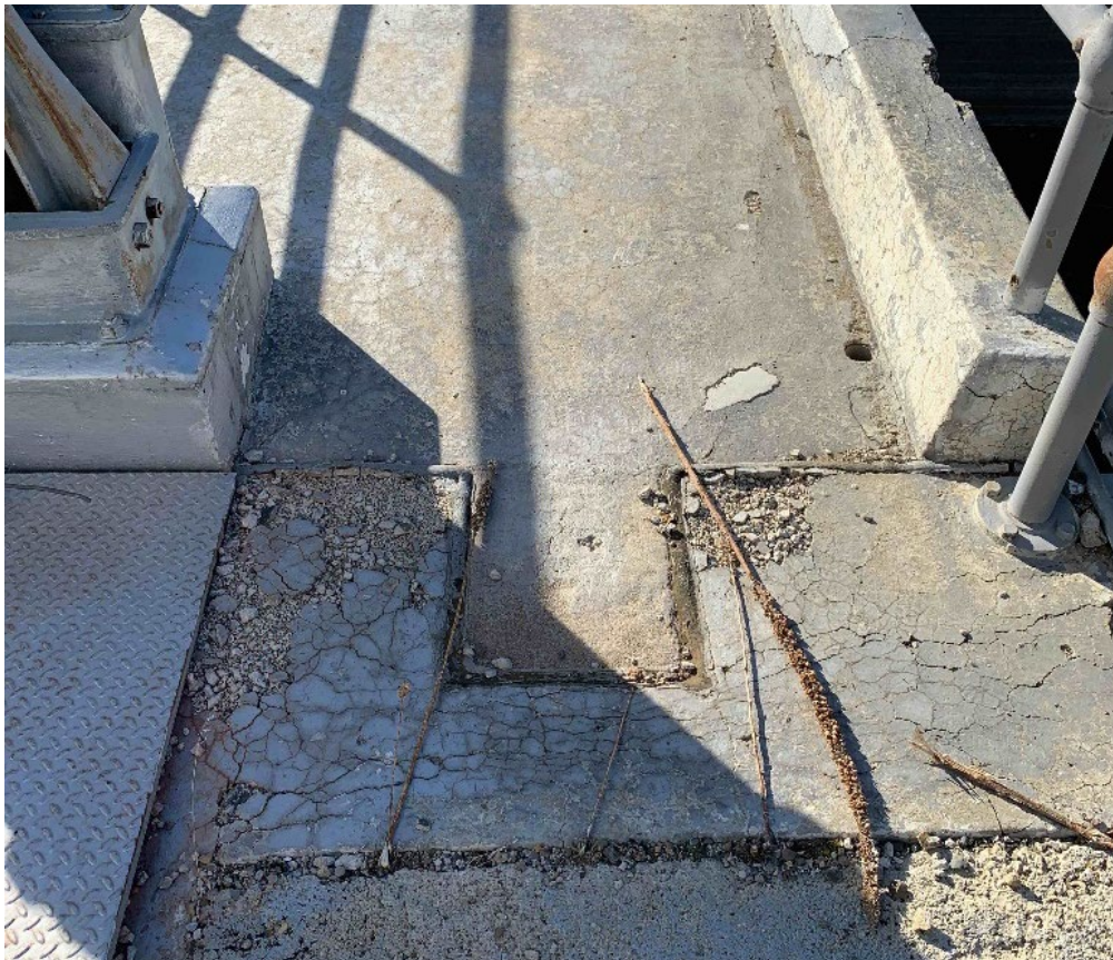
Figure A-6.—Deteriorated concrete on a walkway.
