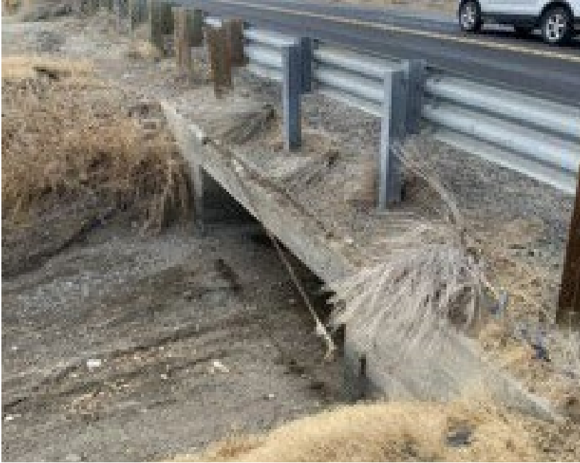
Figure A-1.—Exposed rebar along a bridge crossing over a canal. The bridge is a roadway that has deicing salts applied in the winter. It has not required previous repairs and it is unknown whether concrete corrosion caused the initial concrete deterioration.
