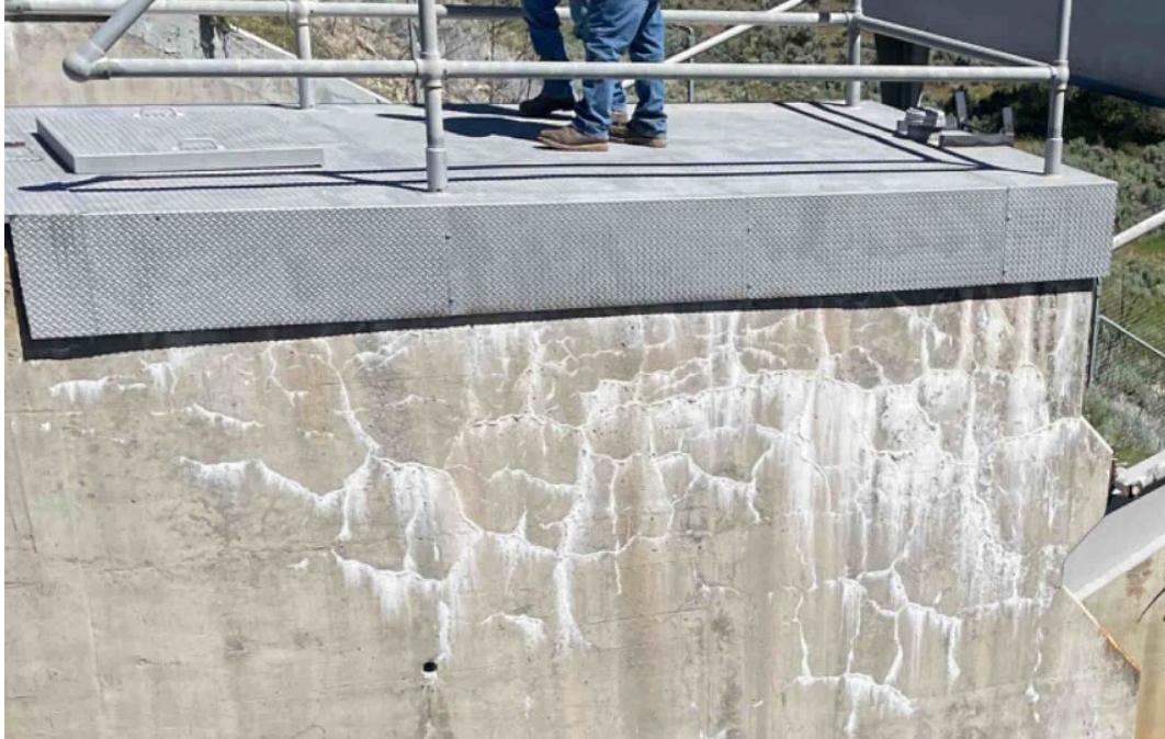
Figure A-7.—Concrete damage, possibly due to ASR. Generally, no corrosion staining is visible, except some possible corrosion staining at the wall on the lower right corner of the image.
