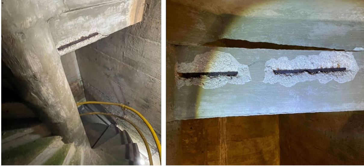
Figure A-5.—Spalling and exposed rebar on underside of stair treads on the spiral staircase between the upper and middle galleries. Rebar corrosion and concrete damage likely due to inadequate cover.
