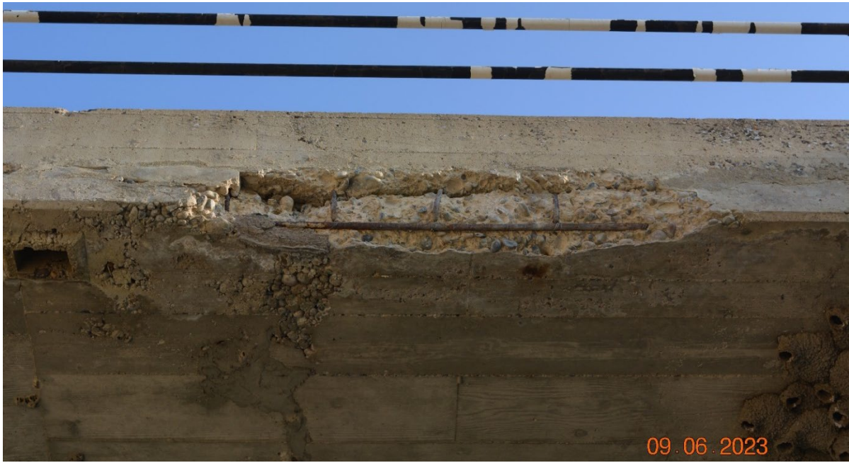
Figure B-3.—Type 1 bridge. Location noted as having cracking, spalling, and one instance of exposed rebar. Corrosion is not explicitly mentioned in inspection reports.
