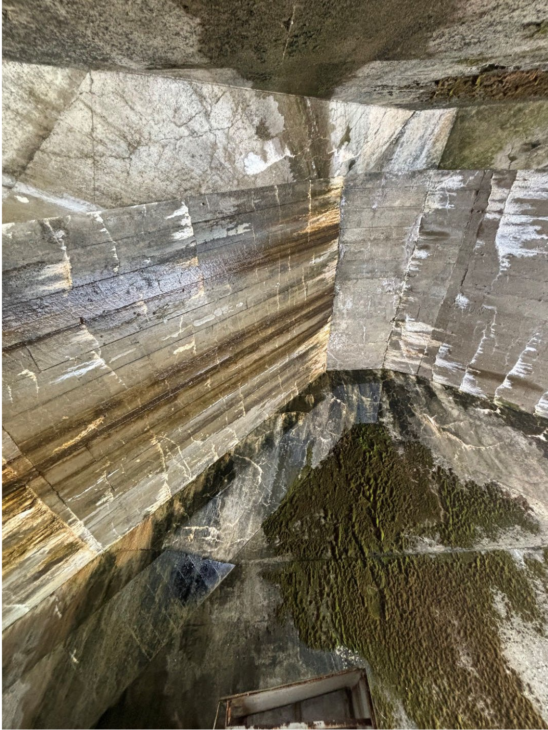
Figure A-9.— Concrete slabs exhibiting widespread horizontal cracking with relatively narrow widths. The source of the cracking is likely due to freezing and thawing.
