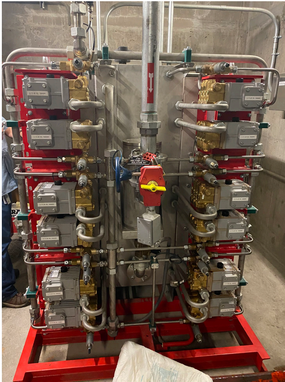
Figure 7. —Example of an electric pump for high-pressure water mist systems.
