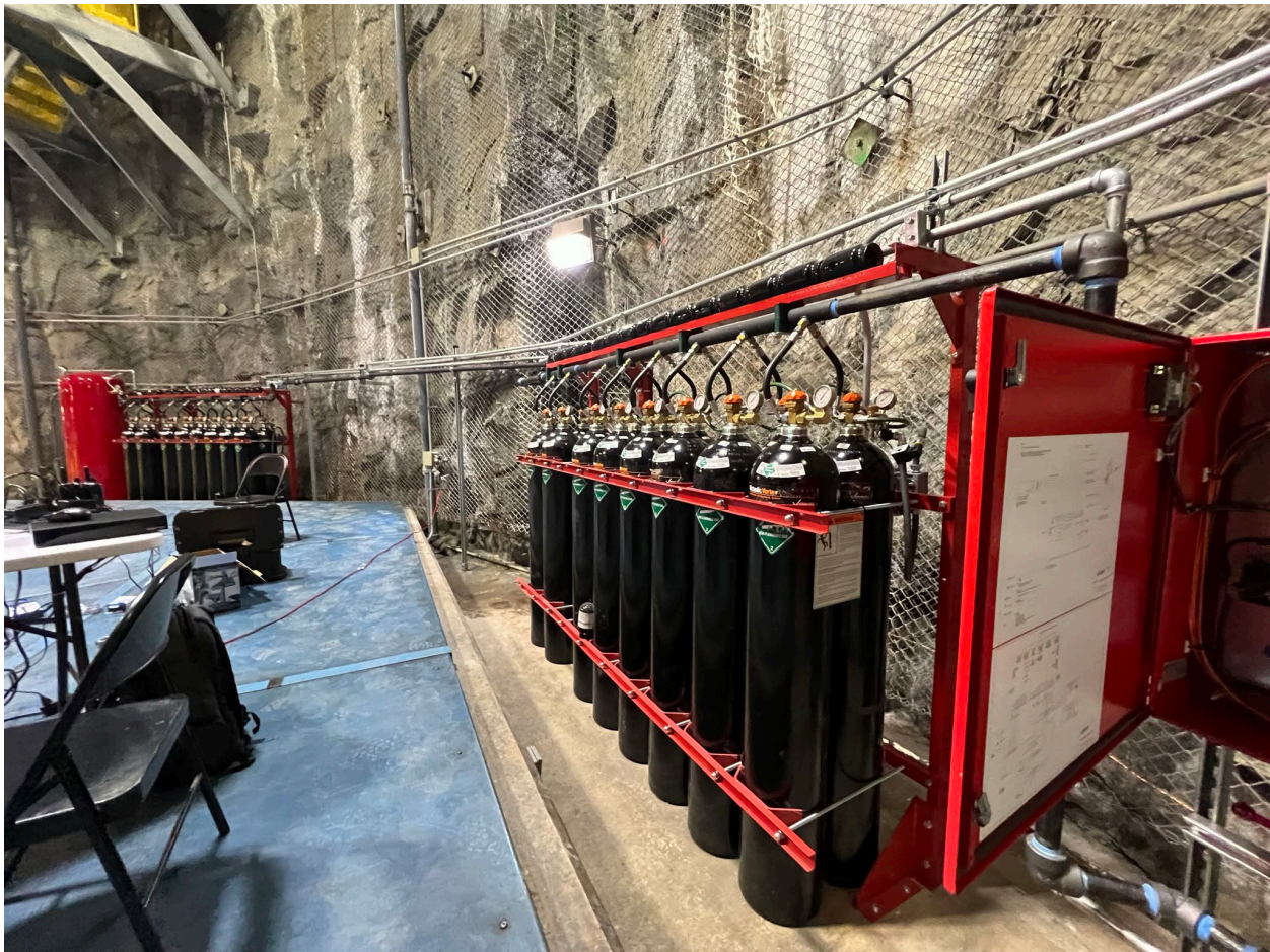
Figure 10. —Hybrid fire extinguishing system used to protect a hydroelectric generator. Photo shows the typical installation with banks of nitrogen tanks connected to a single manifold. The water tank is in the red cylinder in the background.
