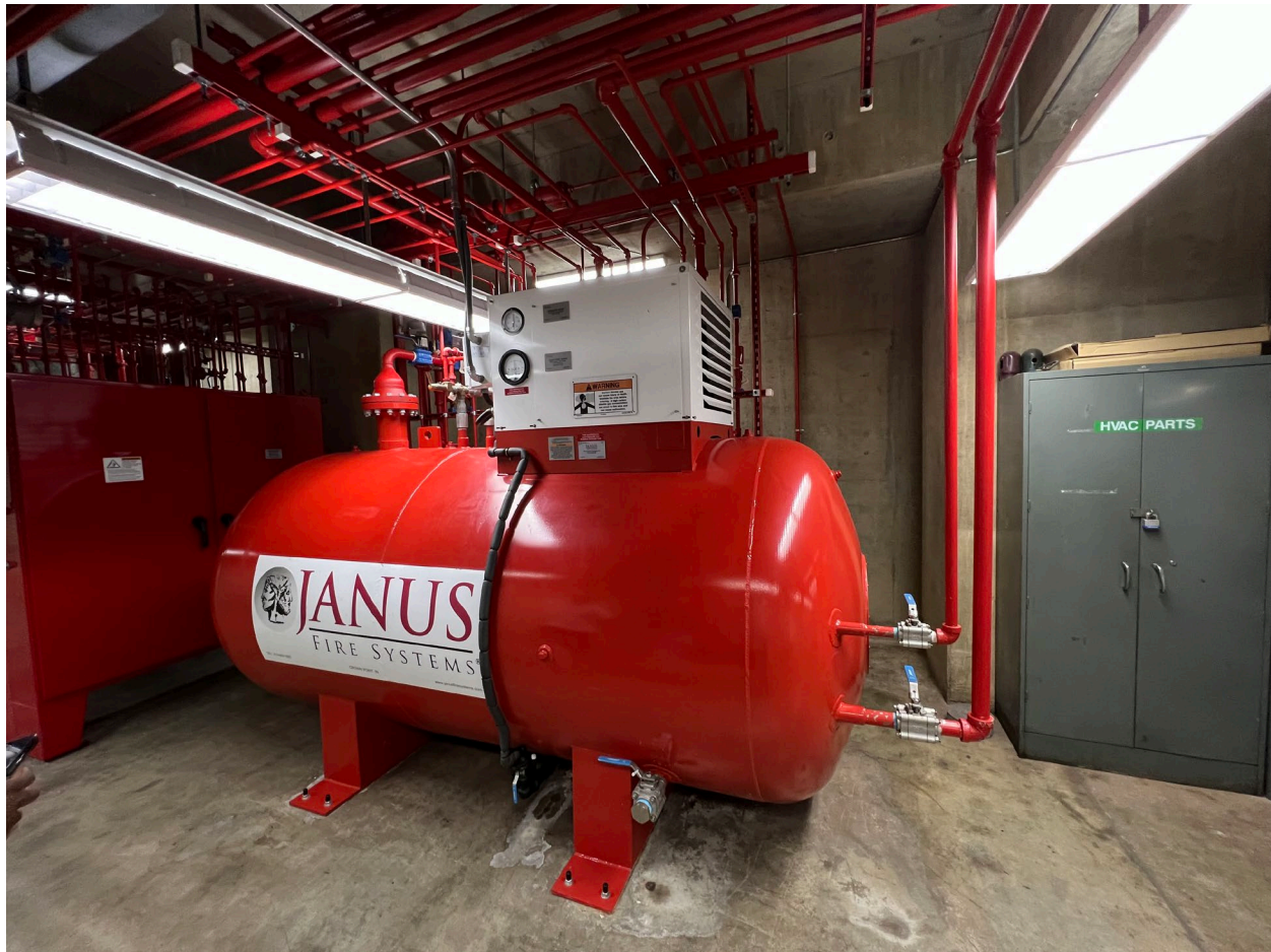
Figure 4. —Typical low-pressure CO 2 system commonly found in Reclamation. A large bulk tank contains all the CO 2 for initial and extended discharge. Routing is in the large red cabinet behind the tank.
