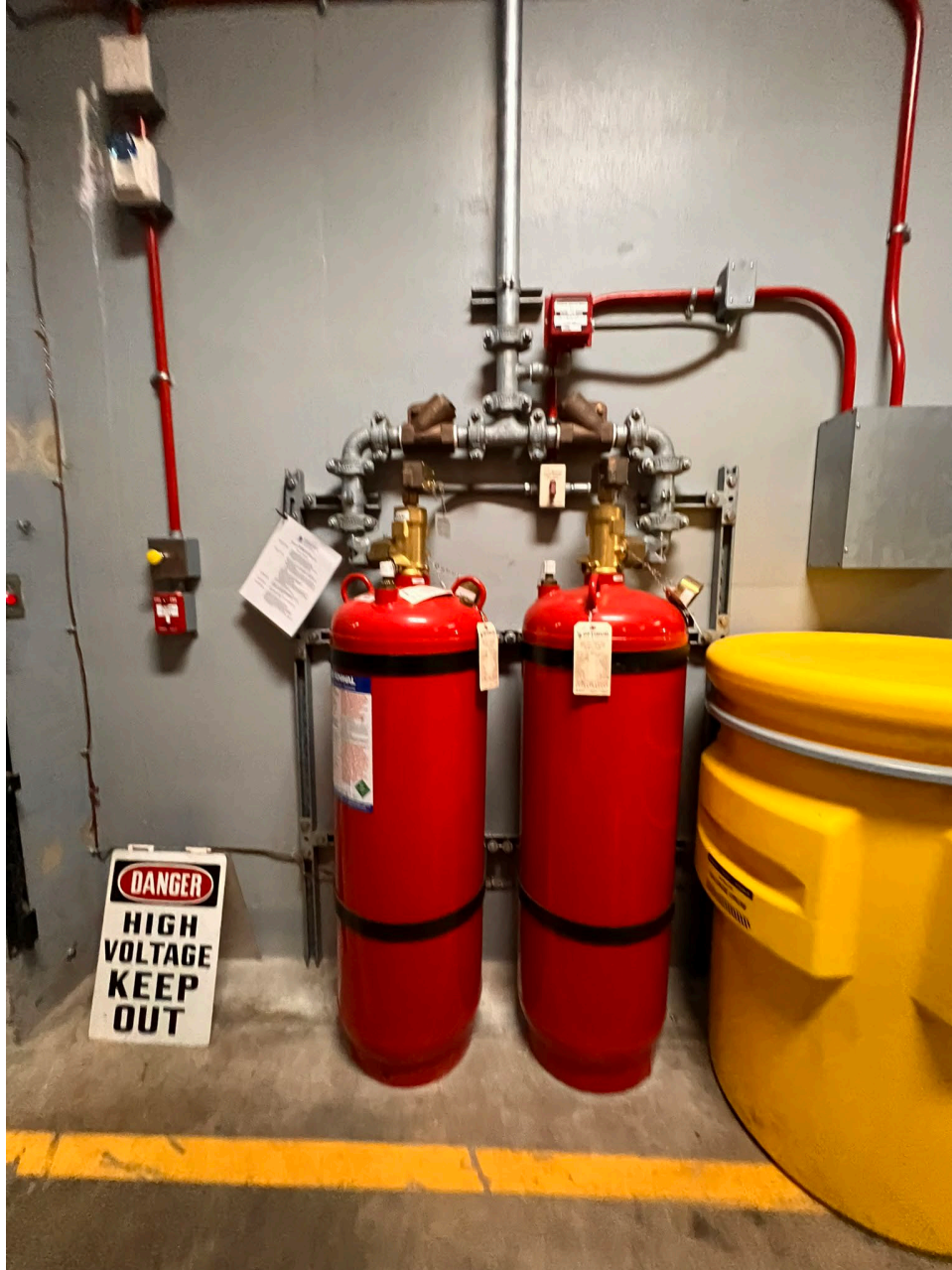
Figure 8. —FM-200 system used to protect an oil storage room in a Reclamation power plant. . The photo shows a typical installation with bulk agent tanks with releasing heads installed on top of the tanks and the piping to the protected space.
