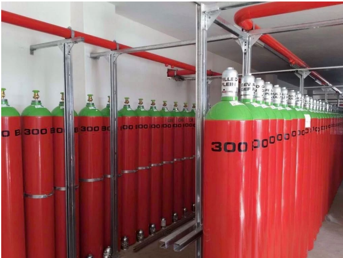
Figure 9. —Typical inert gas system installation. The system shown in the picture is an Inergen gas system recognizable from the green top of the cylinders (FST, n.d.)
