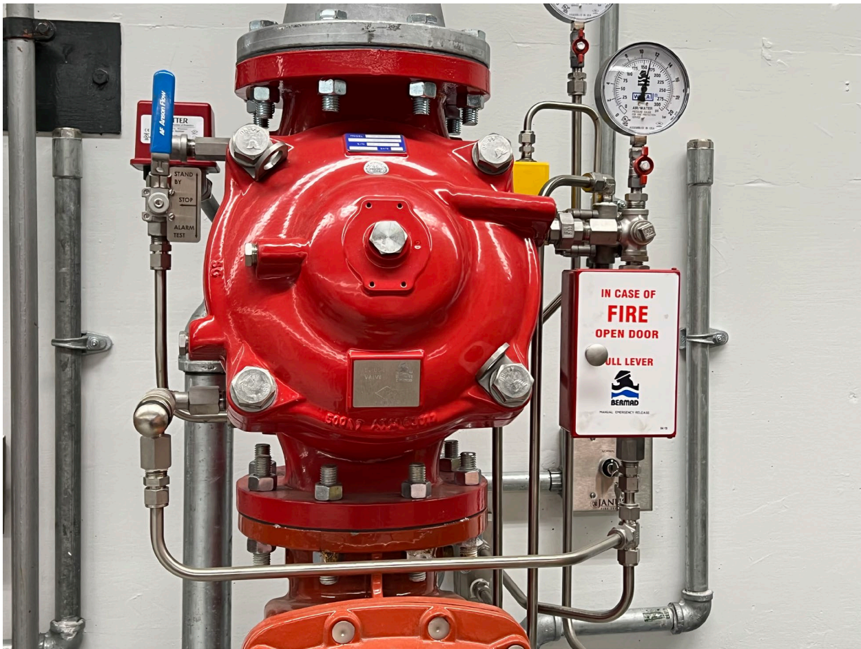
Figure 6. —Typical pre-action deluge valve for water spray systems This system uses an electronic solenoid to initiate the system pneumatically. The photo also shows the manual override switch.
