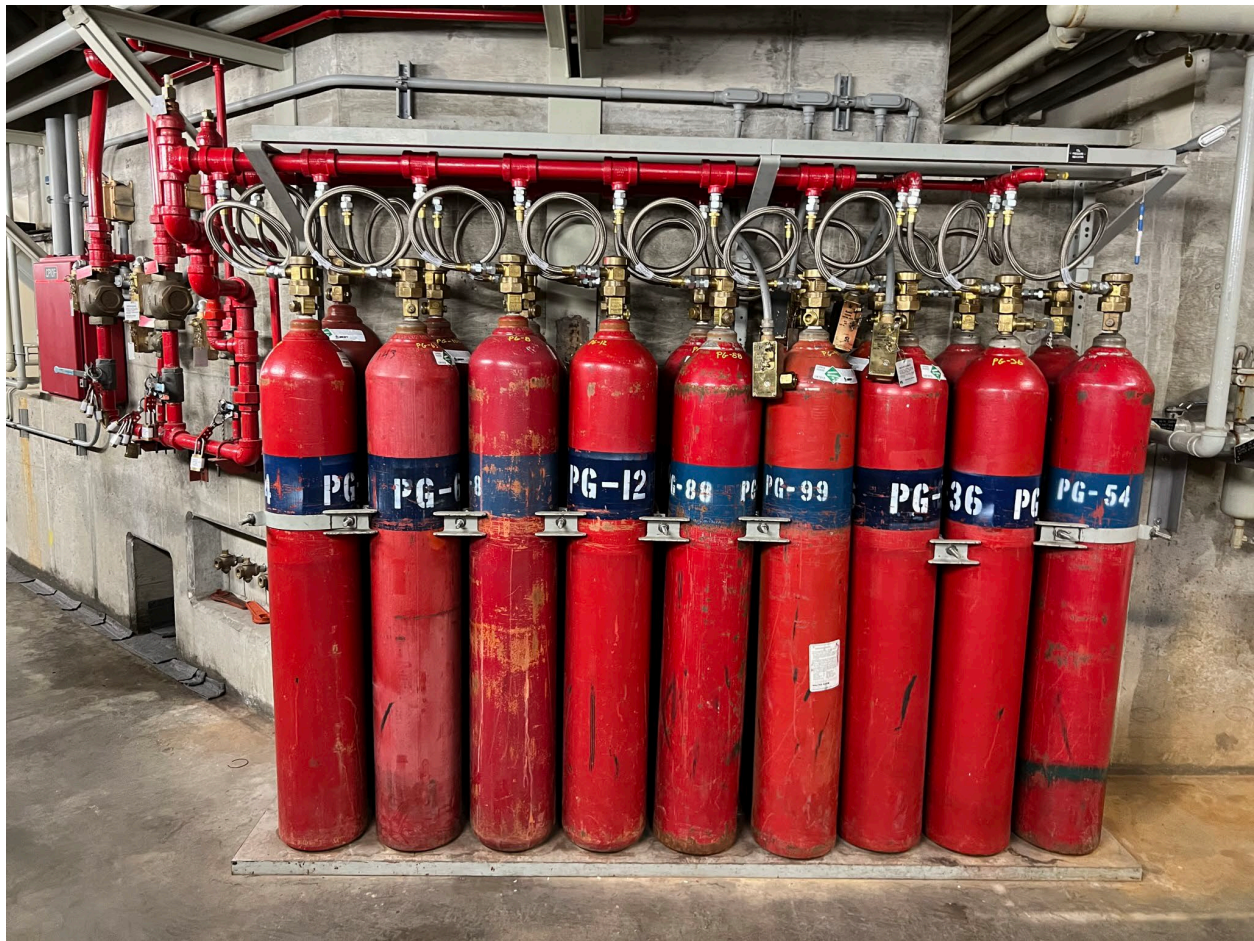
Figure 1. —Typical high-pressure CO 2 system commonly found in Reclamation.
