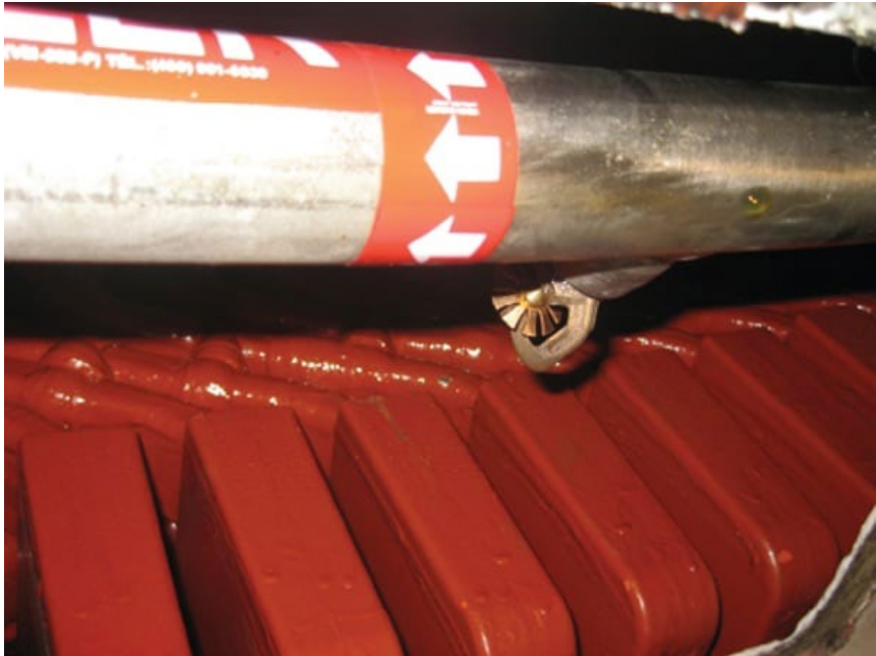
Figure 5. —An automatic sprinkler head on a pre-action system inside an air-cooled generator. The sprinkler head is shown installed directly above the stator coils. (Dieken, 2011).
