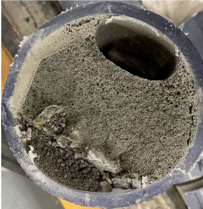
Photograph 26.—PLDCC specimen from 8-foot horizontal-debris, with air void and lower density at top, and partially encapsulated coarse and fine aggregate debris at bottom.
