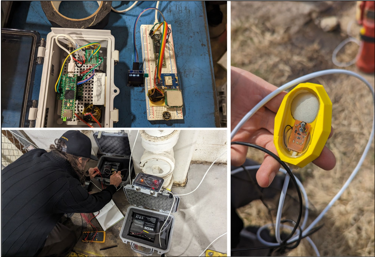
Figure 23.—Various photos of the prototype data logger and piezoelectric sensor taken during the initial water release test at GSA Facilities Building 810.
